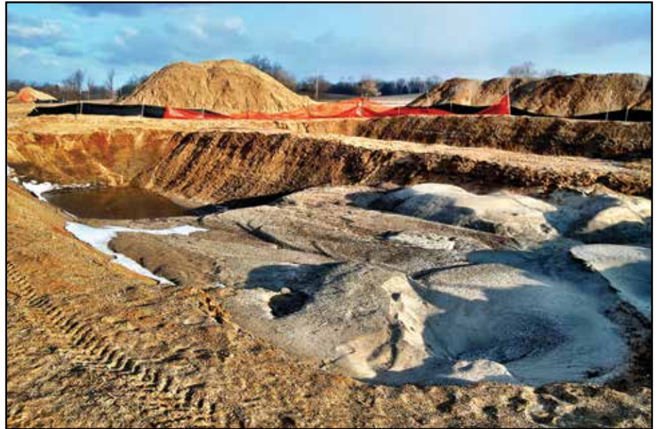
The material removed using the Sand Wand™ is pumped to discharge or dewatering pits. These pits are temporary and excavated in upland areas.
