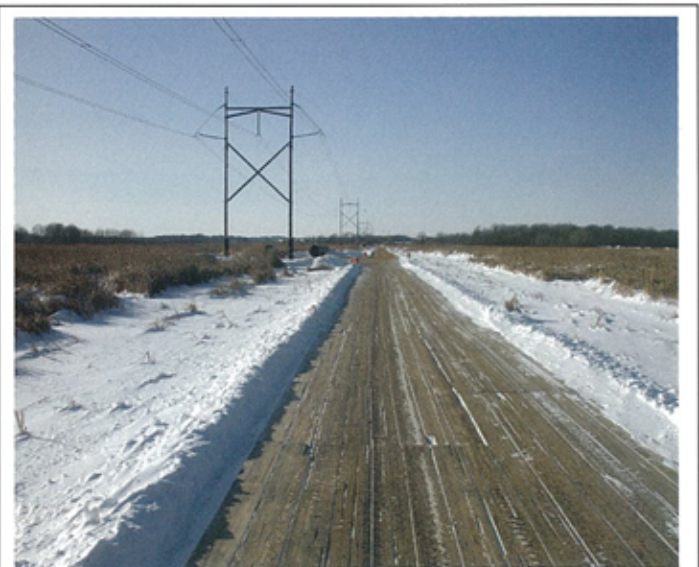
The Bear Creek Marsh wetlands access solution incorporated RFID-GPS technology in each mat to ensure no non-native materials were left on the site after construction completion. The completed temporary access road is used year-round; a special eco-friendly snow-removal product keeps the surface ice-free, even during tough Wisconsin winters.
