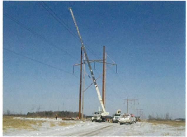
After erecting the two individual weathering steel poles, ATC contractor crews are in the process of lifting the crossarm in place. When complete the crossarm will support the electrical conductors. The average weight of each fully assembled steel H-frame structure is about 14,000 lbs.
