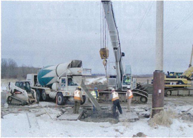
ATC contractor crews are pouring concrete into a recently excavated foundation cavity. Steel reinforcement bars and anchor bolts were positioned in the hole for embedment in the concrete. About 3,500 cubic yards of concrete was used throughout the project.
