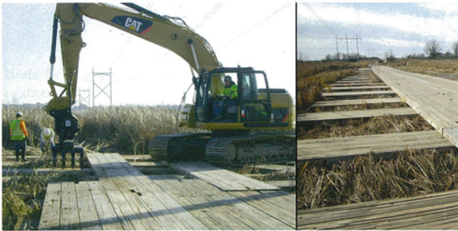
An excavator is used to lay road deck surface on top of floating foundation mats. Environmental protection required that equipment could not be taken into any part of the wetland. The supports and bridge were laid one segment at a time. Then equipment was driven on that new bridge section to work on the next bridge segment.
